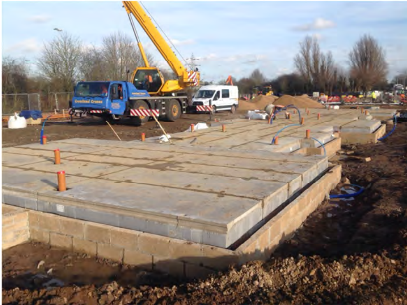
Ground works start on Lynnsport 4 and 5 sites of the major housing development
