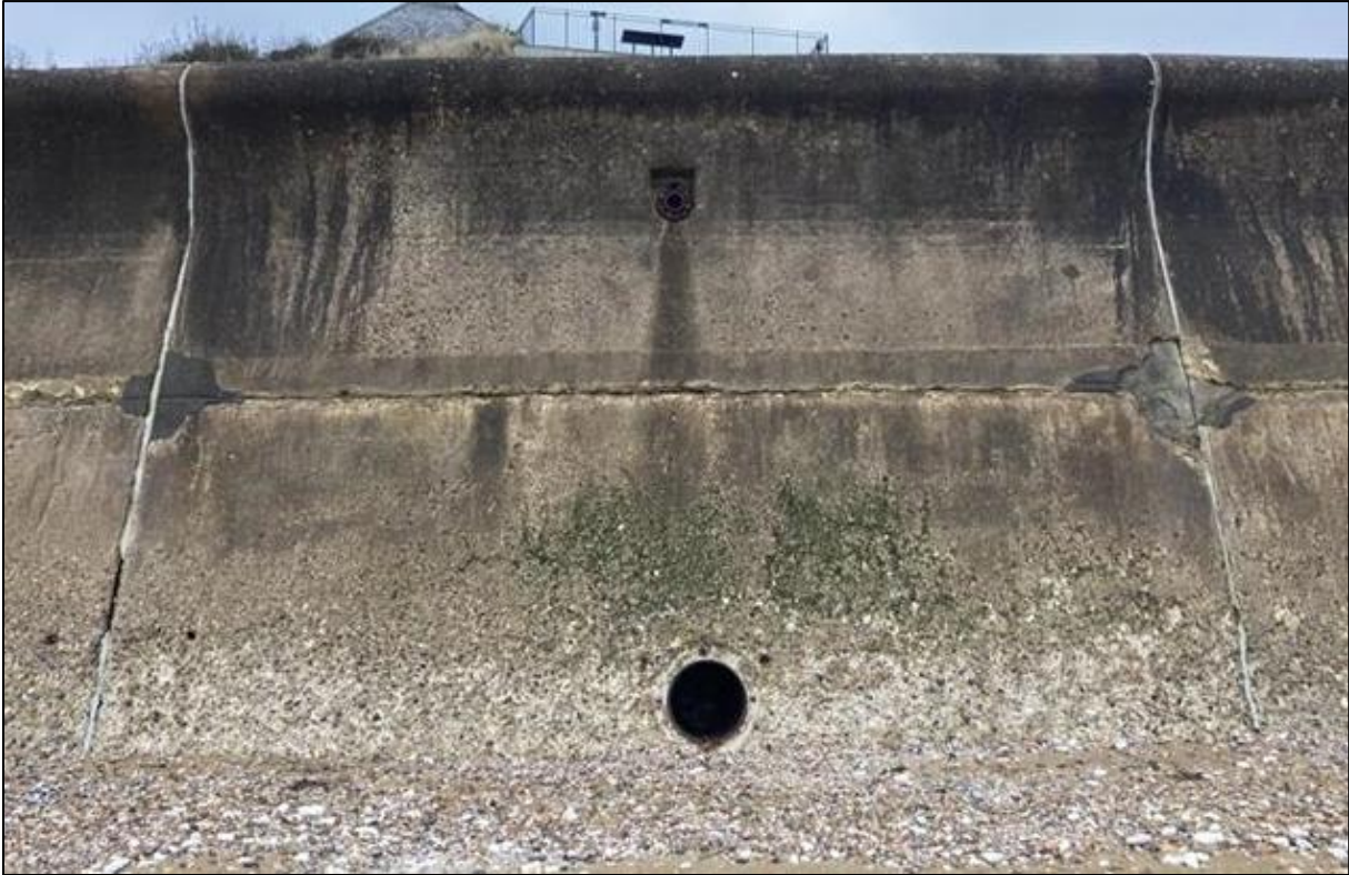
Missing redundant outfall cover before
