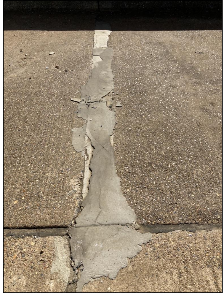
Concrete patch repair required on promenade
