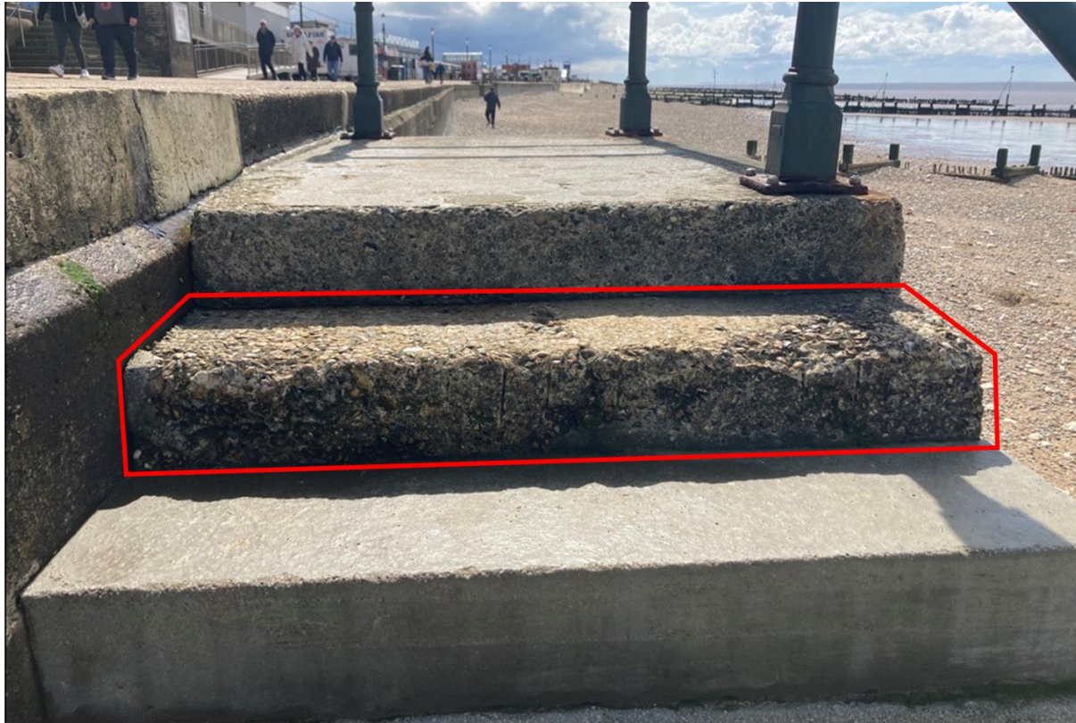
Concrete repair (re-casting) required to beach access step
