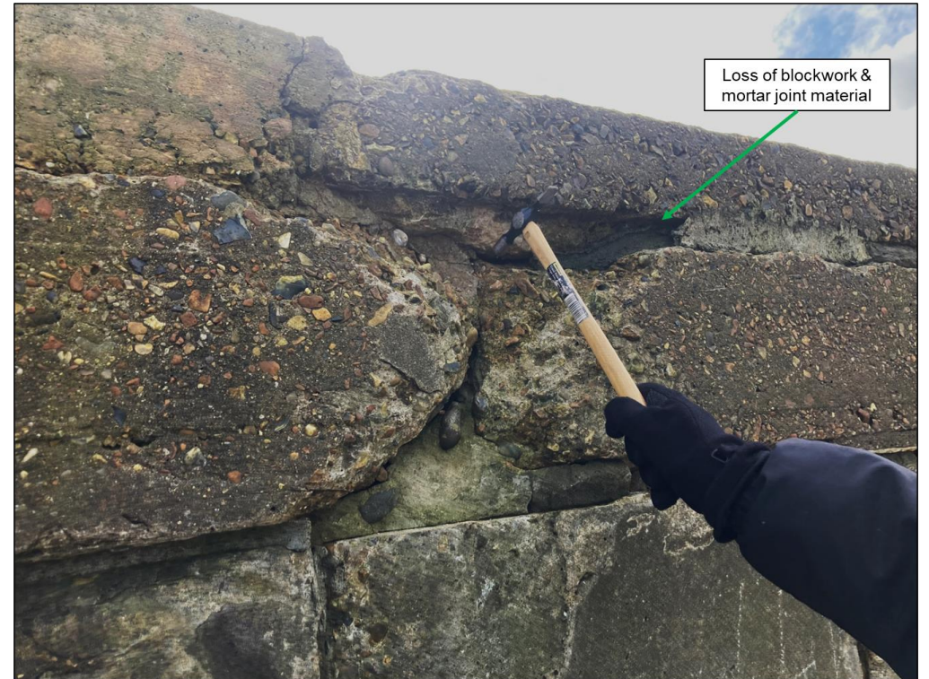
Concrete repair required to blockwork seawall
