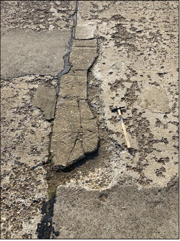
Promenade condition prior to temp patch repair.
