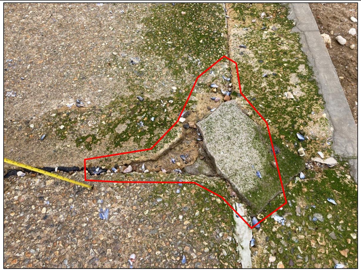
Concrete patch repair required to slipway
