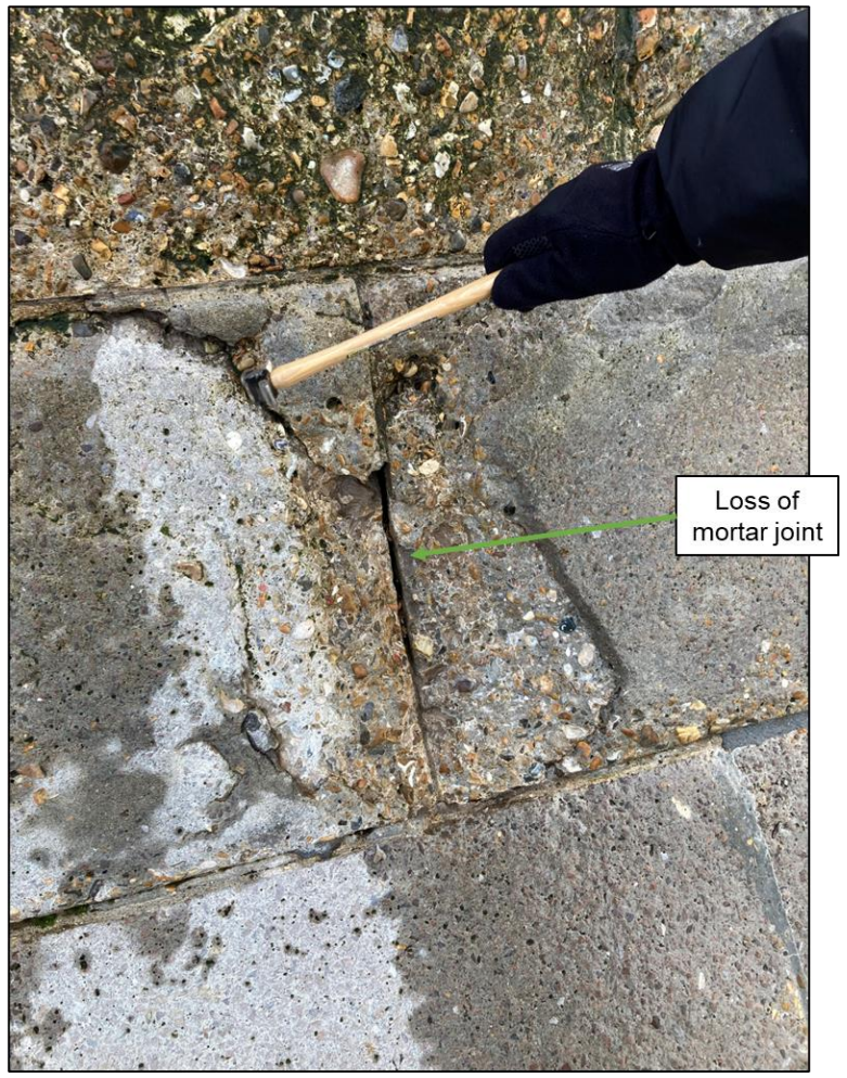
Replacement of mortar joint required on blockwork seawall
