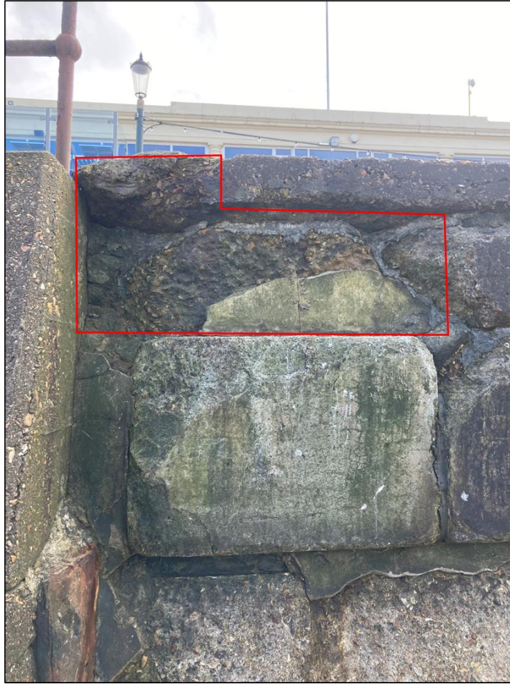
Concrete repair required to blockwork seawall
