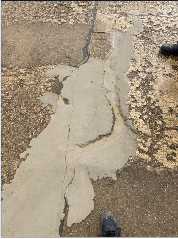
Current promenade condition with temporary repair
