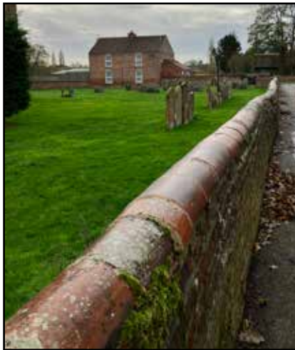
F.51: Historic wall with curved capping surrounding St. Peter's Church. (Photo © AECOM 2022)
